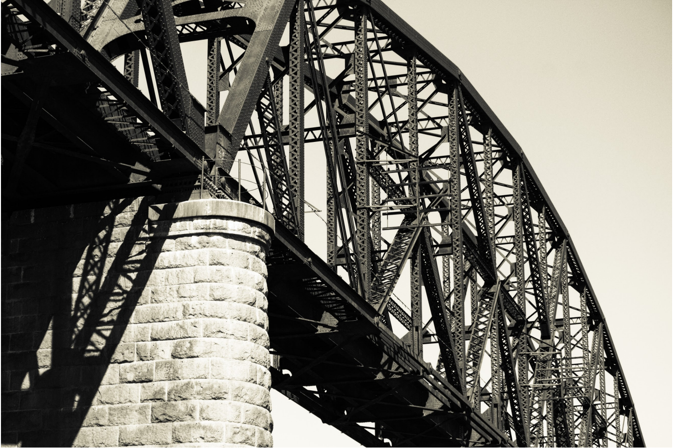
Photo taken by Charles Metz of the Liberty Memorial Bridge in Burleigh County, North Dakota.
